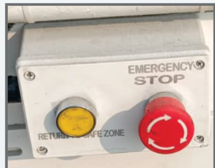
Emergency Stop in Bucket
